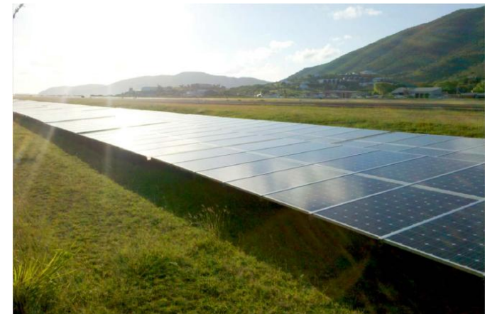
Cyril E. King Airport on St. Thomas (451 kW Capacity)
